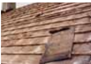
Building structure degradation: mould and mildew.
